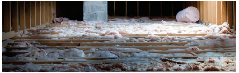
Installing loft insulation is just one simple way to increase the energy efficiency of any home
