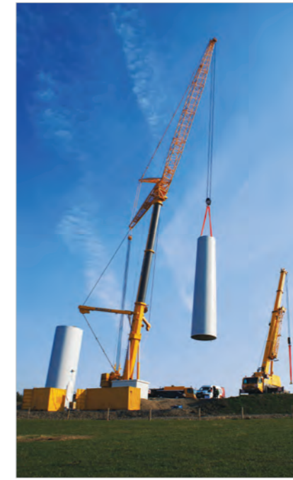
Construction of 100m to tip height turbine at West Durham Wind Farm
